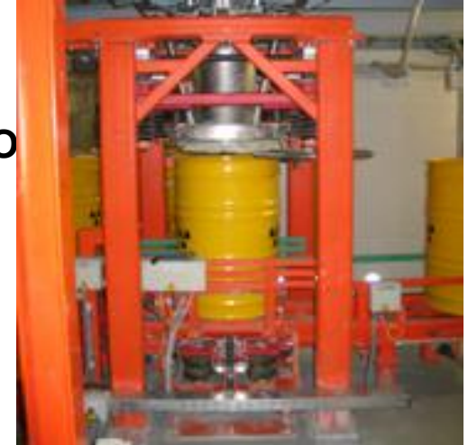
Drum Filling Station
